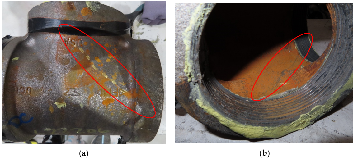
Figure 12. Post Disassembly Tee Fitting Body Rupture Images: (a) Body Rupture Outside of Fitting; (b) Body Rupture Inside of Fitting.
