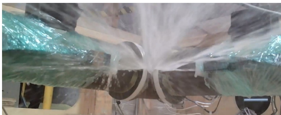
Figure 9. Elbow Fitting Rupture Observed from Lab.
