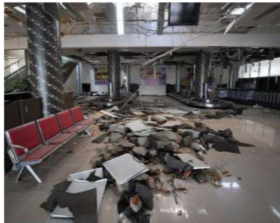
Figure 1. Non-Structural Damage that Occurred in the 2018 Palu Earthquake.
