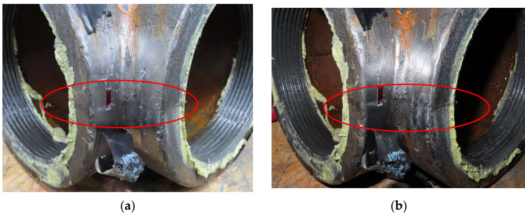
Figure 13. Post Disassembly Tee Fitting Casting Line Rupture Images: (a) Casting Line Tee Rupture 1; (b) Casting Line Tee Rupture 2.
