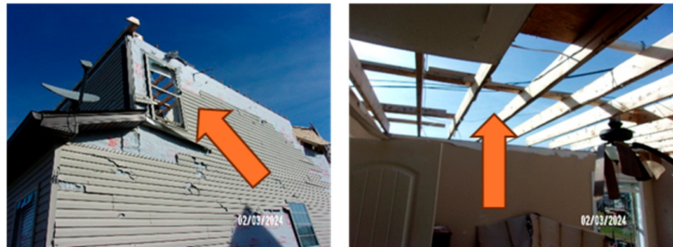
Figure 3. (Left): Damage to the windward window. (Right): Damage to the roof panels.
