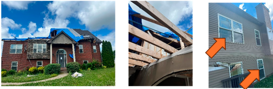
Figure 11. Case study 3: (Left) and (Center): Roof damage. (Right): Blown-out windows.
