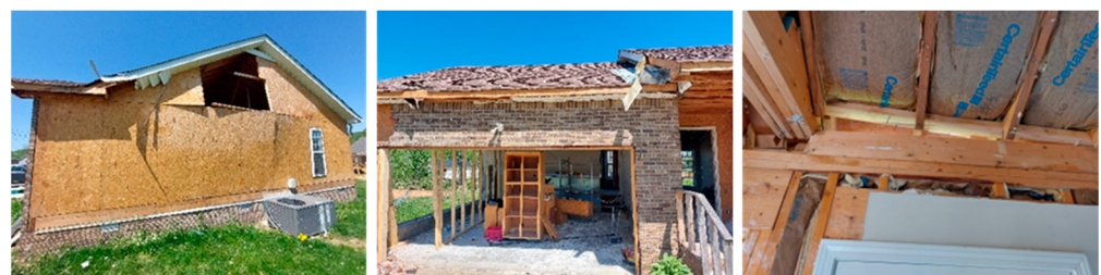
Figure 7. Case study 2: Damage to the front garage door, the adjacent wall, and the gable-end wall.
