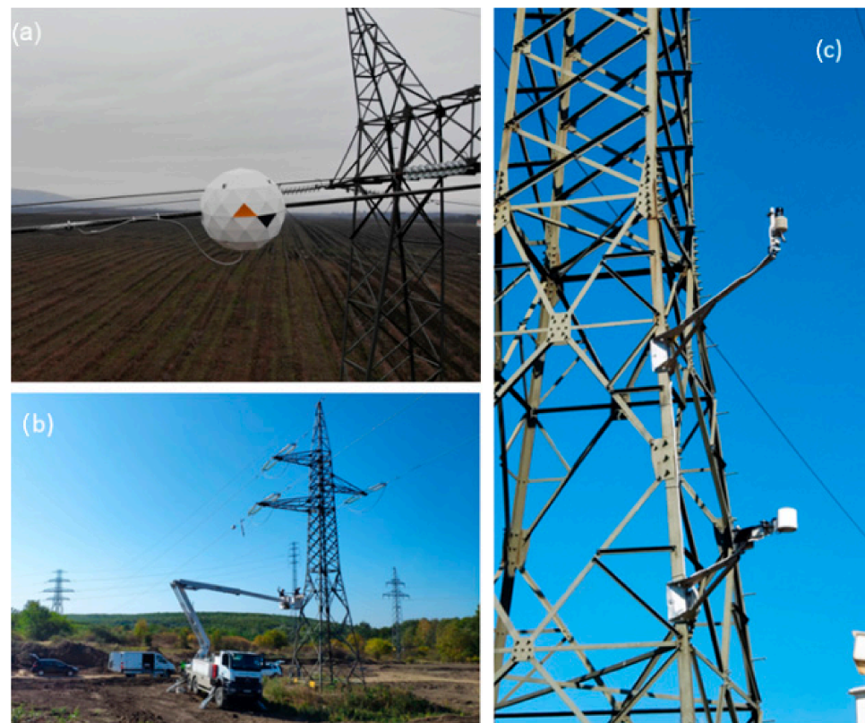
Figure 1. Installation of dynamic line rating equipment in the Hungarian distribution and transmission system: (a) line monitoring sensor, (b) weather station, (c) weather station.
