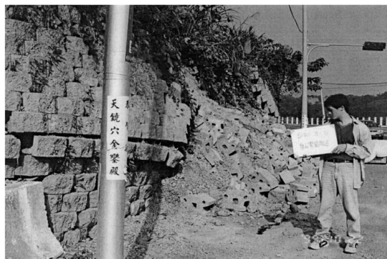
Figure 3. Severely damaged GRS-MB at Site 1 [23].
