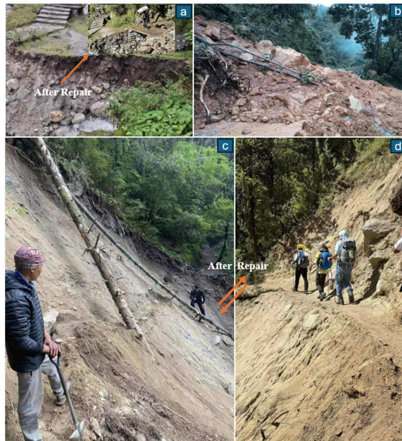
Figure A4. The Namche Jorsalle landslides (5 October 2025). (a) After repair and before repair condition of the trekking route of first landslide; (b) the second landslide; (c,d) after the route was reopened after repair and maintenance (14 October 2025). Source: [139,140], and Adhikari Madhav/Everest Base Camp Trek Information Centre.
