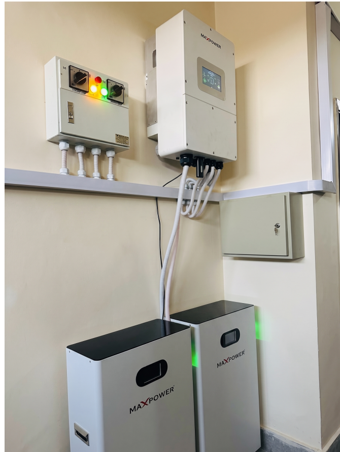
Figure 3. MAXPower inverter, protection enclosure and associated battery-storage hardware at the monitored Lahore PV plant.
