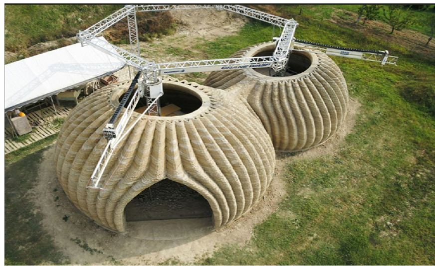
Figure 1. The WASP Crane system Arrangement © WASP.
