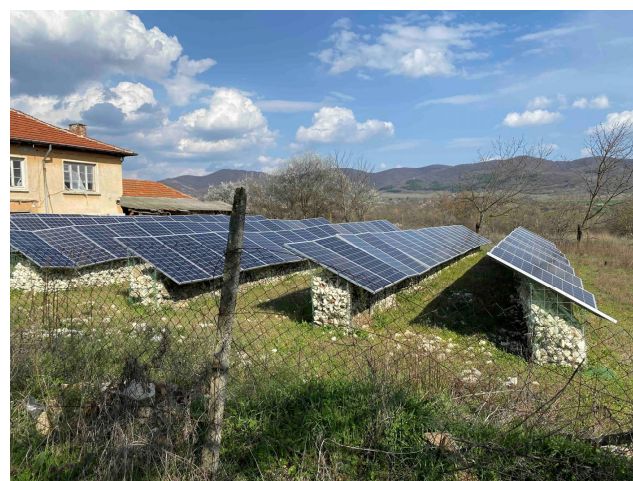
Figure 6. Suboptimal installation leading to direct loss of productivity from panel misalignment; very unstable during wind events and shading from ground foliage shades the entire system.
