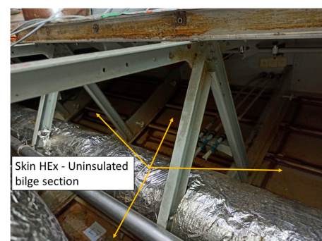
Figure 3. Bilge skin heat exchanger.
