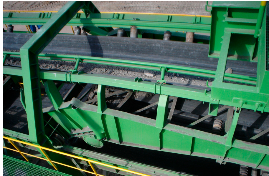
Figure 1. Belt conveyor failure due to buckling phenomena.
