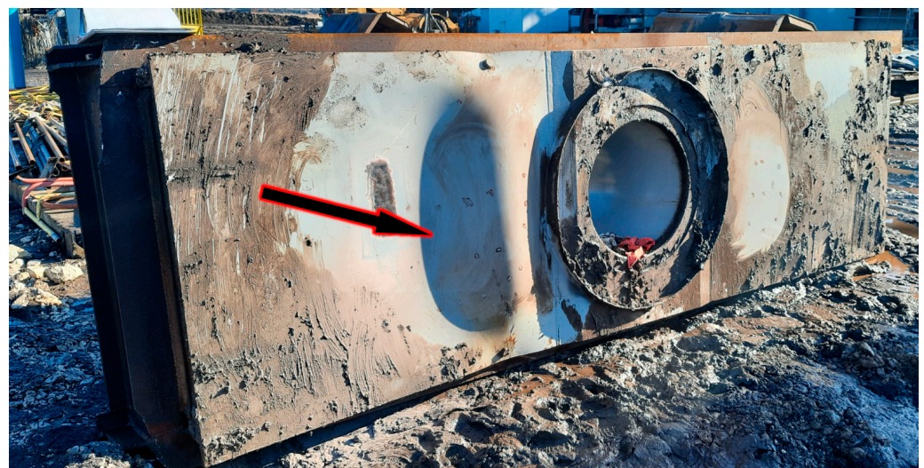
Figure 5. The rotating support girder after disassembly. The buckling area is marked with a black-red arrow.
