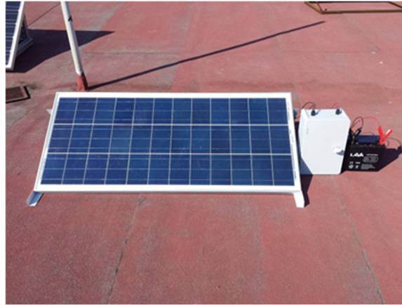
Figure 1. Installed photovoltaic system.
