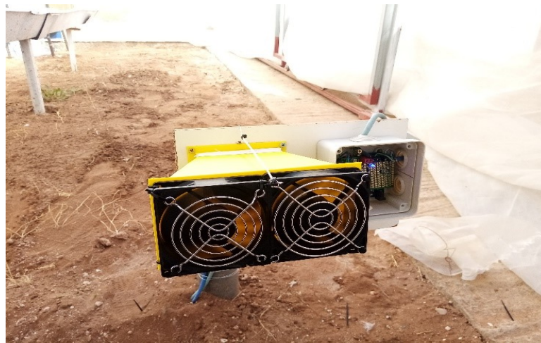
Figure 6. Experimental setup for the installation of airflow regulation and measurement techniques.
