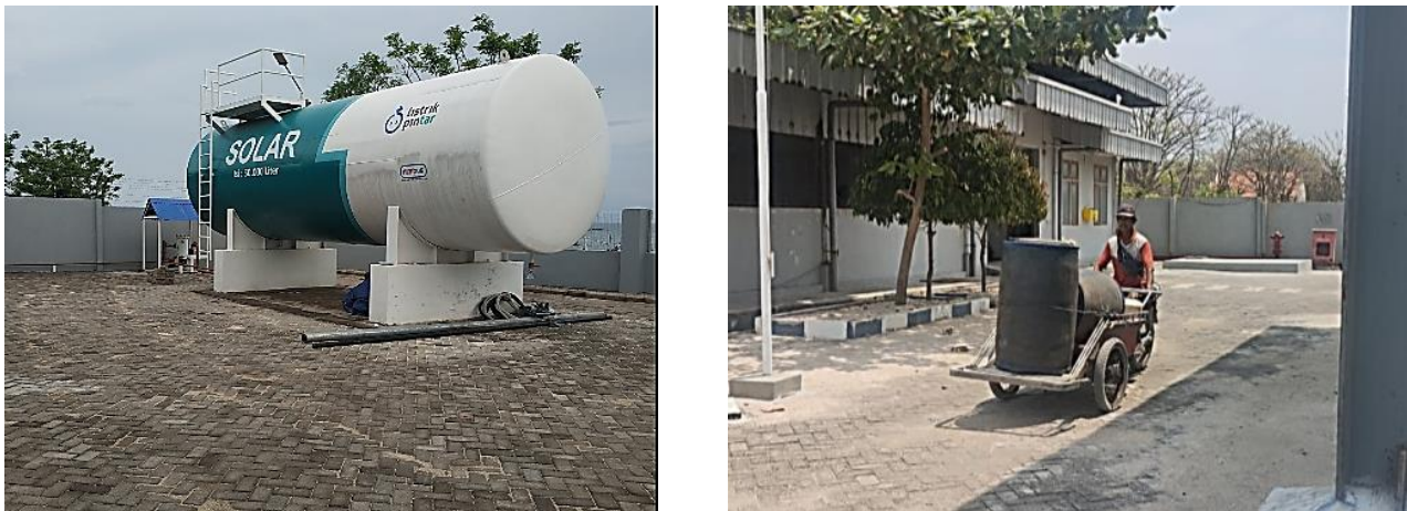
Figure 7. The Diesel Power Plant on Gili Ketapang.
