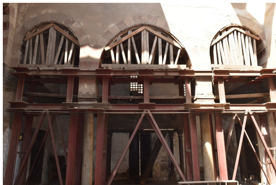
Figure 2. Example of historic monument in Old Cairo, after the 1992 earthquake. Photo by the authors.
