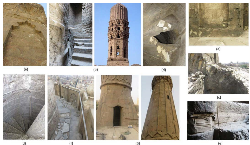
Figure 14. Examples of structural vulnerability studies of historic masonry minarets in Old Cairo. Adapted from [49] under the terms and conditions of a CC BY 4.0 agreement. Different patterns of deterioration found in (a) the uppermost part of the Ibn Tulun minaret; (b) the body and the upper part
