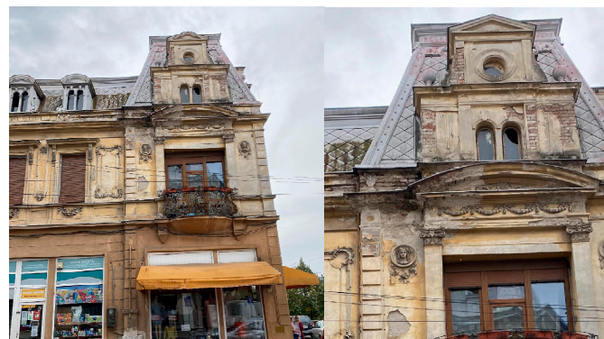
Figure 10. The Haberehn Palace moderate deterioration. The picture was taken in 2021.
