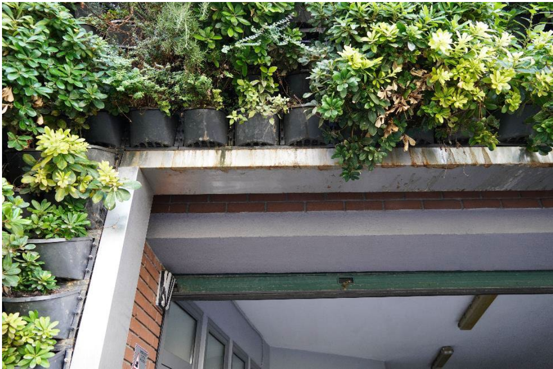
Figure 5. Corrosion phenomena of a metal infrastructure in the building of the Directorate of Urban Environment Management of the Municipality of Thessaloniki, Thessaloniki, Greece.
