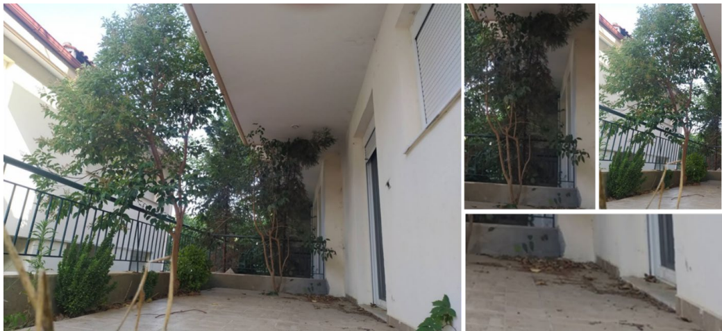
Figure 6. Distorted growth of trees and bio-debris at a planted balcony in Thessaloniki, Greece.
