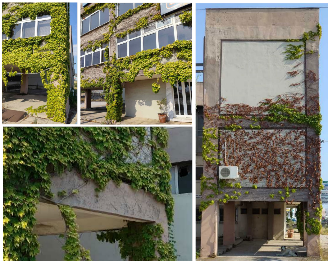
Figure 4. Green façade on a company’s building in Thessaloniki with recorded damages on vegetation and the building’s envelope.
