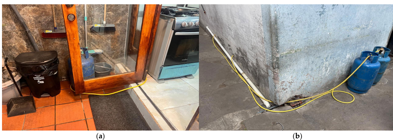
Figure 6. Observed conditions of flexible LPG connections: (a) hose passing under a door; (b) excessive hose length.
