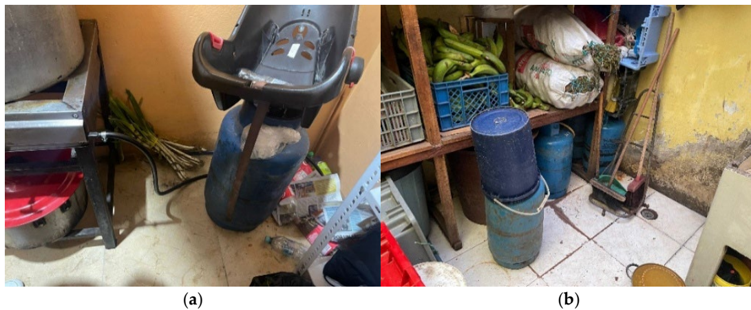
Figure 3. (a) Cylinders are placed too close to combustible materials; (b) restricted accessibility to LPG cylinders.
