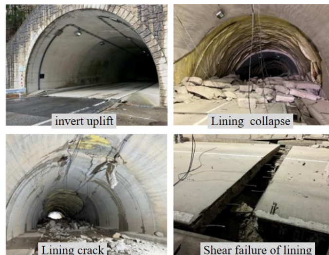
Figure 1. Diverse seismic damage modes (invert uplift, lining collapse, lining crack, shear failure of lining) reproduced from Damage Analysis of Tunnels during the 2024 Noto Peninsula Earthquake, Ministry of Land, Infrastructure, Transport and Tourism (MLIT), 2024 [1].
