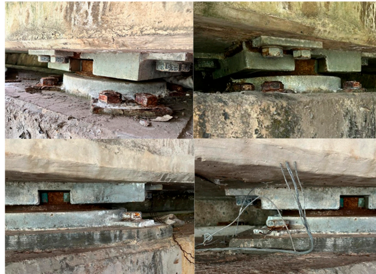
Figure 14. Support mechanisms of the southern pier, showing surface oxidation due to rainwater.
