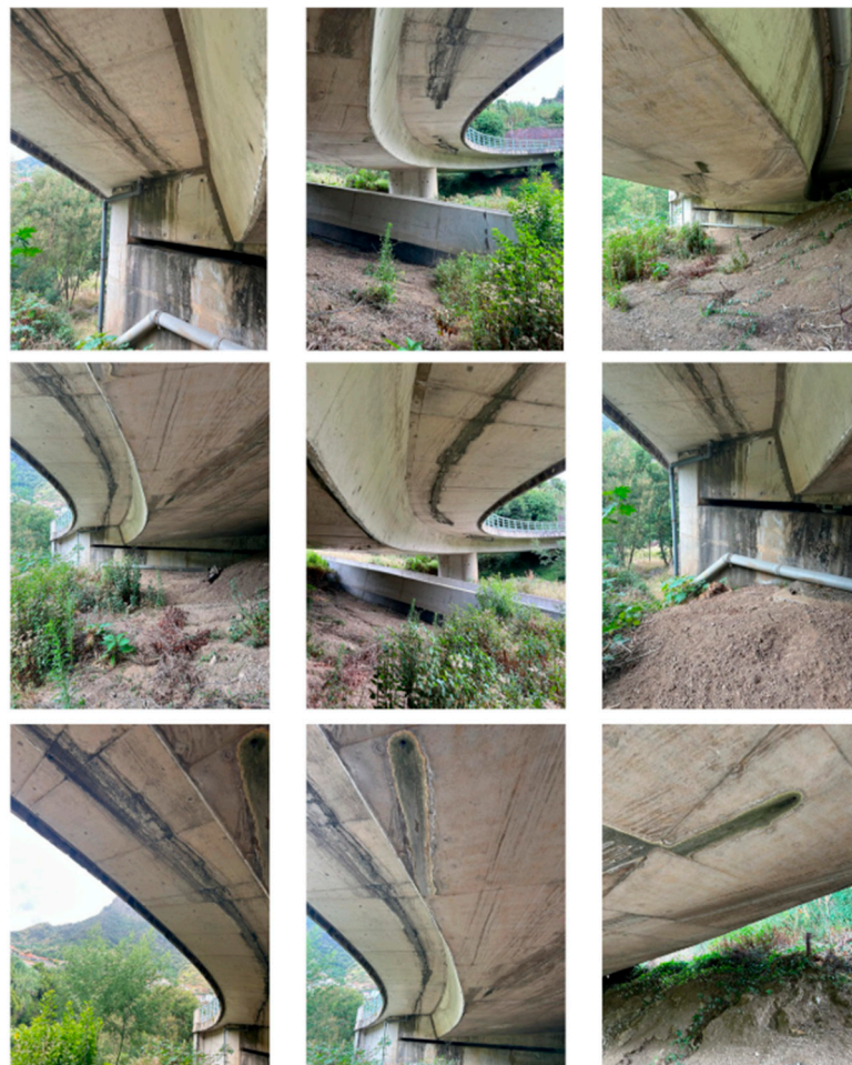
Figure 15. Rainwater runoff on the bridge deck, viewed from below, southern Ribeira do Junçal area.
