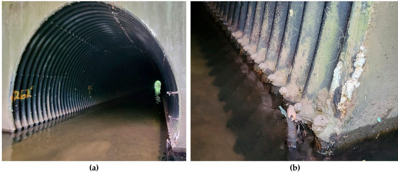
Figure 1. (a) In-service CMP culvert; (b) sediment build-up at the culvert waterline.
