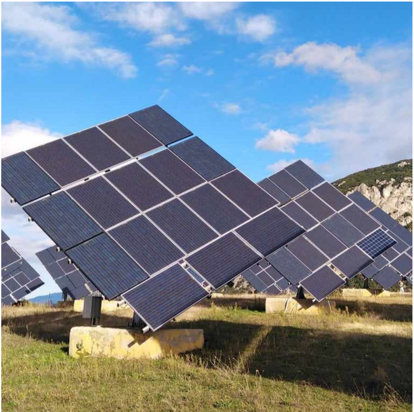
Figure 8. Picture of the solar park that is the focus of this case study.
