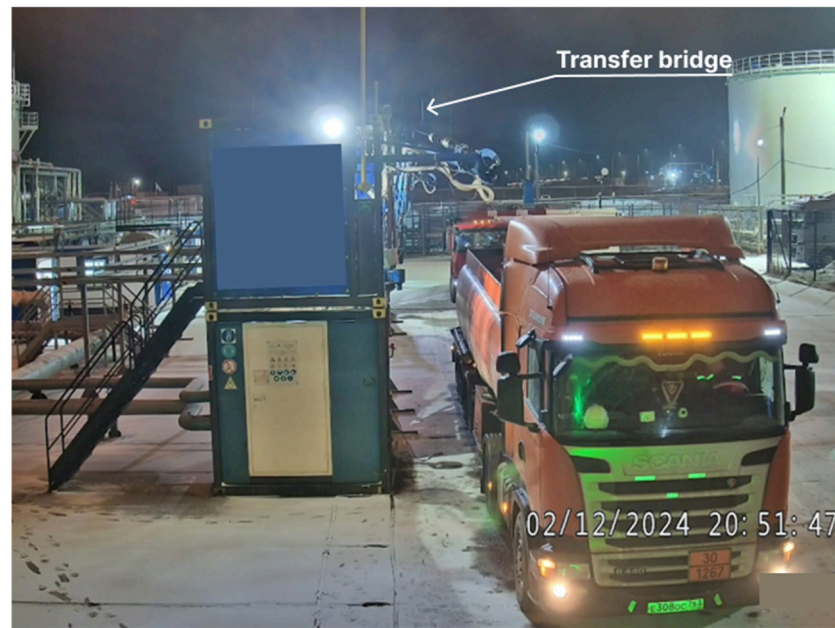
Figure 10. The site of the automated filling system at night.
