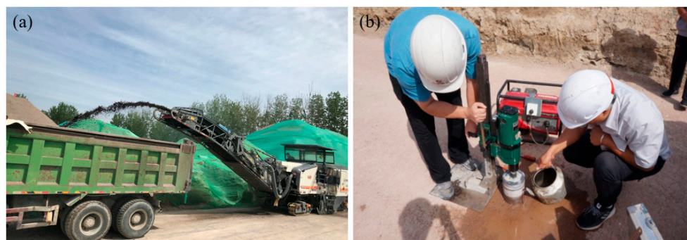
Figure 20. Schematic of core drilling and sampling process. (a) Pavement milling; (b) Core drilling and sampling.
