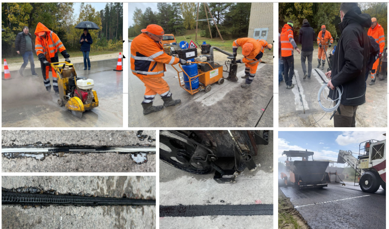
Figure 10. Temperature FBG and distributed strain sensor integration in road pavement layer.
