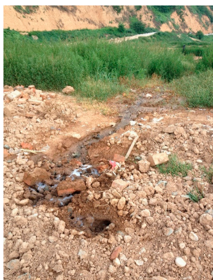
Figure 9. Leachate leakage points.
