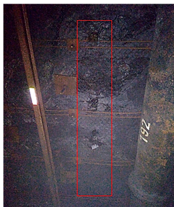
Figure 13. Photographs of expansion holes in the field.
