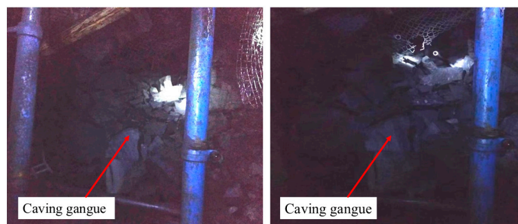
Figure 14. Top slab collapse at the end of the roadway.
