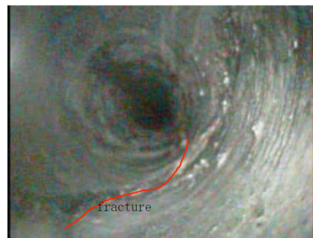
Longitudinal crack at 27.15 m of measuring hole
