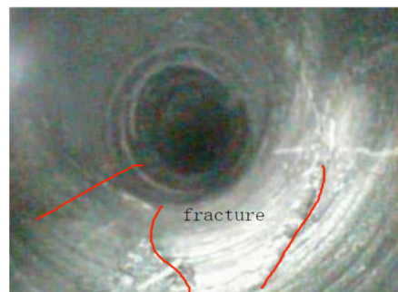
Longitudinal crack at 22.68 m of measuring hole
