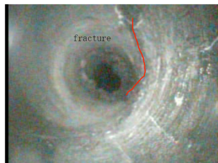
Longitudinal crack at 34.58 m of measuring hole
