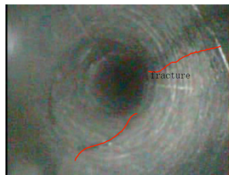
Longitudinal crack at 35.54 m of measuring hole
