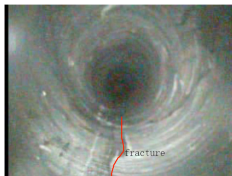
Longitudinal crack at 19.08 m of measuring hole
