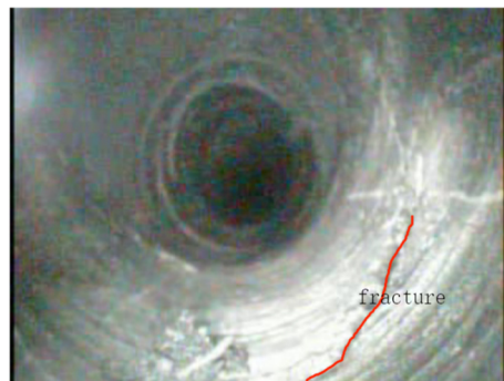
Transverse crack at 14.86 m of the measuring hole
