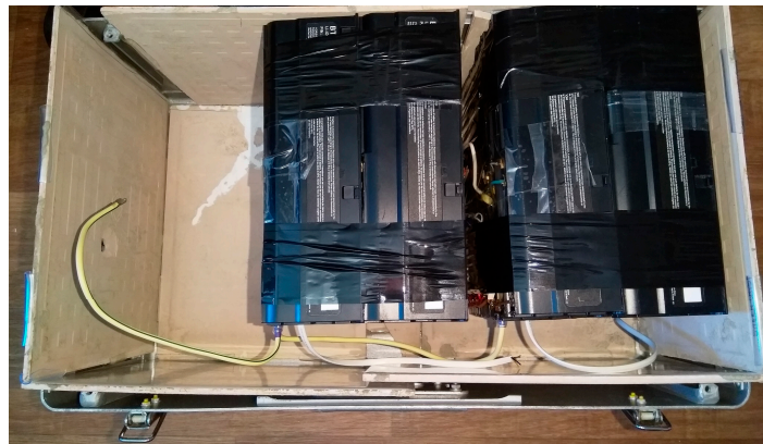
Figure 12. Creation of 27s lithium-ion package to obtain the accumulator compatible with the proposed voltage range and to simplify verification of the work of the created 96 V inverter in a wider voltage range.
