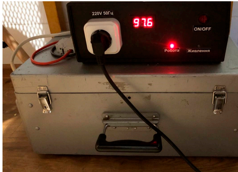
Figure 16. This is the normal operating of the inverter with the connected fridge.
