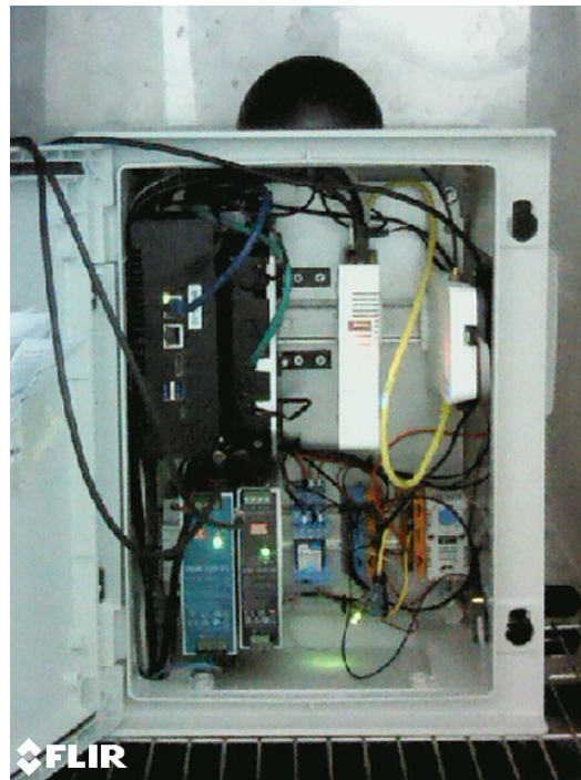
Figure 1. Internal view of the enclosure.
