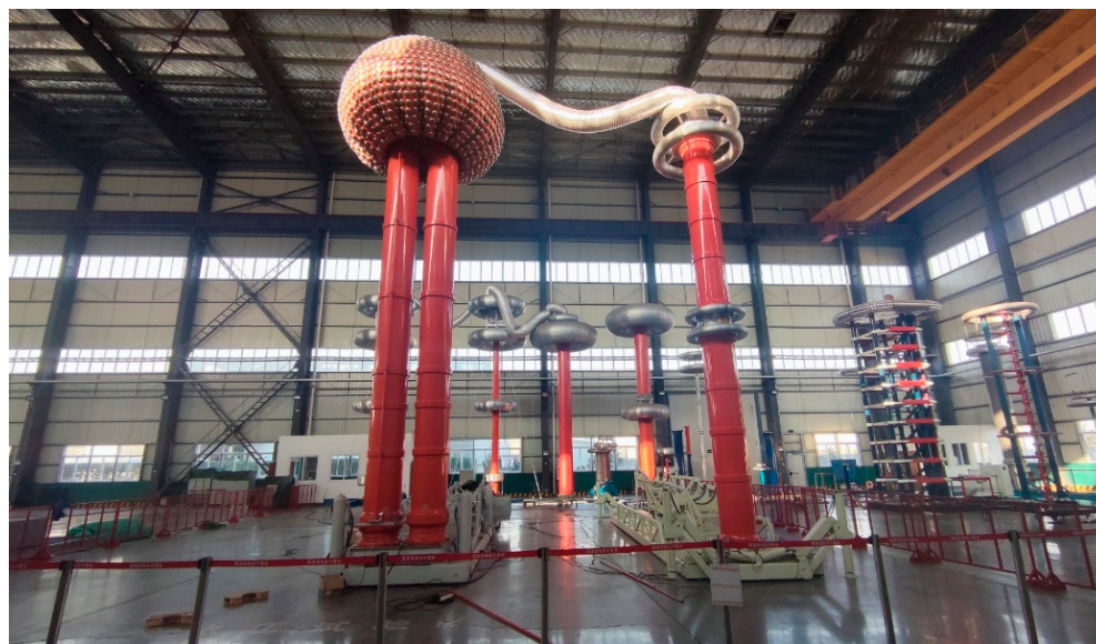
Figure 11. Experimental platform for insulation resistance measurement at 550 kV.
