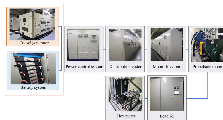
Figure 5. Test bed for testing proposed generator-battery hybrid system.
