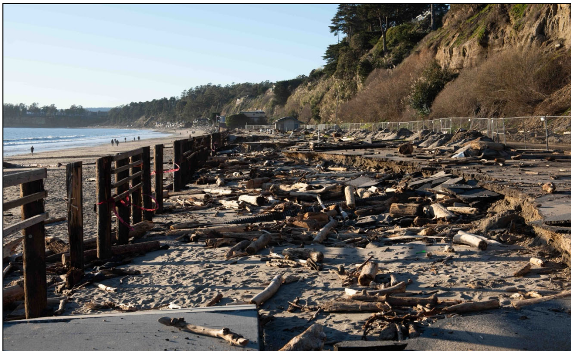
Figure 5. Destruction of timber bulkhead and former back beach RV parking area at Seacliff State Beach on 5 January 2023 (Kim Steinhardt).
