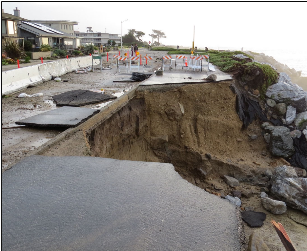
Figure 3. Wave overtopping of the bluff along West Cliff Drive in the city of Santa Cruz on 5 January 2023 led to erosion of weak upper bluff materials, collapse of several sections of the pedestrian pathway, and threats to the roadway (Photo by Author).
