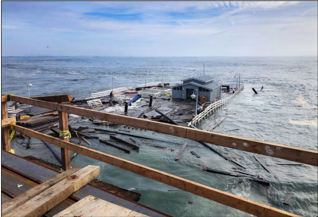
Figure 9. The outer end of the Santa Cruz Municipal Pier after collapsing into the ocean on 23 December 2024 (Brad Porter, City of Santa Cruz).
