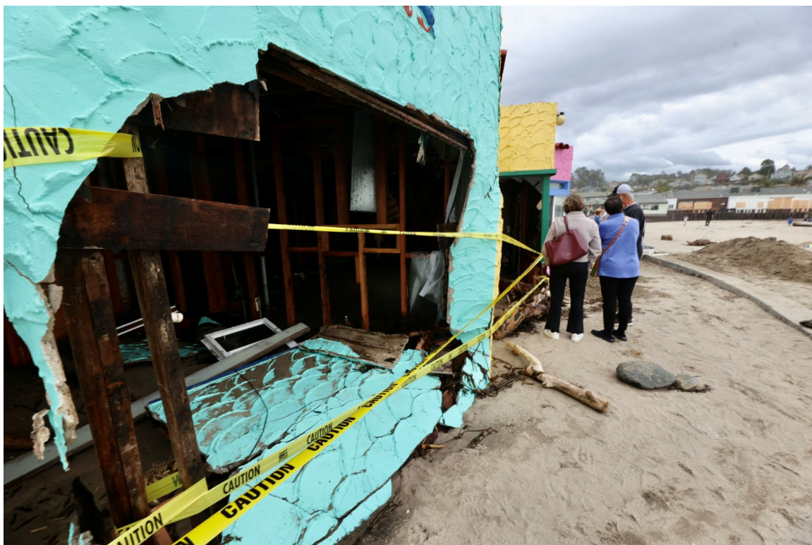
Figure 6. 2 January 2024, damage to beach-level cottages as waves and debris broke through exterior walls (Kevin Painchaud—Lookout Santa Cruz).
