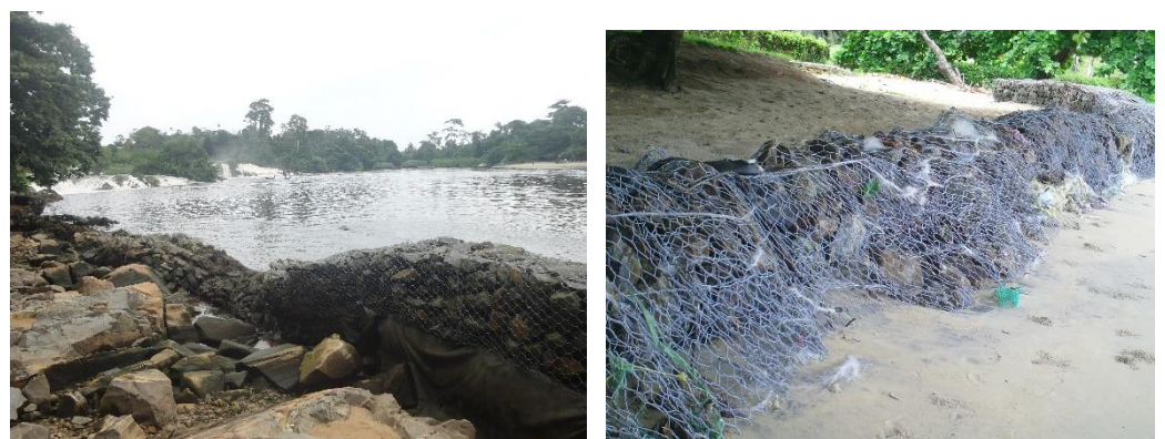
Figure 19. Gabions or cords of rockfill and sandbags at Lobe Falls and Ebodje. Rockfill berms are one of the most common measures for stabilizing the coastline. However, this is a mixed success with the rising sea currents (source: Tchindjang, 2017–2019).
