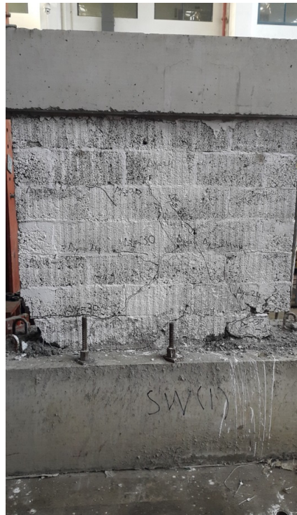
Figure 11. End-of-test picture of entire specimen SW1.
