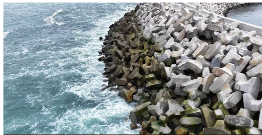
Figure 2. Current Condition of the Main Breakwater at Chancay Port (Photographed on 27 August 2025, depicting the turning point of the main breakwater indicated by the white arrow in Figure 1b).
