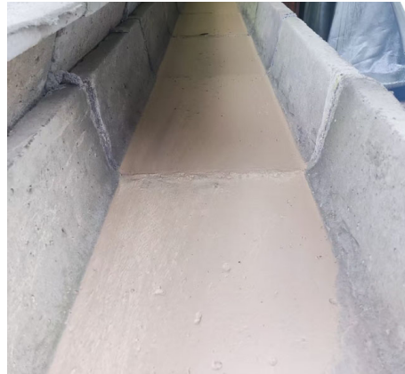
Figure 12. Full-Scale Test View of Sediment Accumulation in Rectangular Drainage Trench with 1% Slope.
