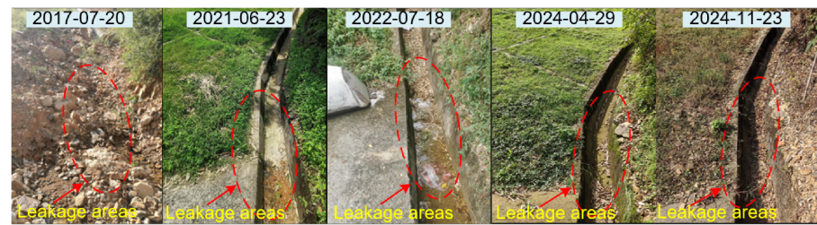
Figure 12. Photographs showing the change in dam slope leakage before and after grouting treatment.
