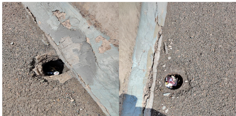
Figure A6. Disease observation of drainpipe and diversion tank.
