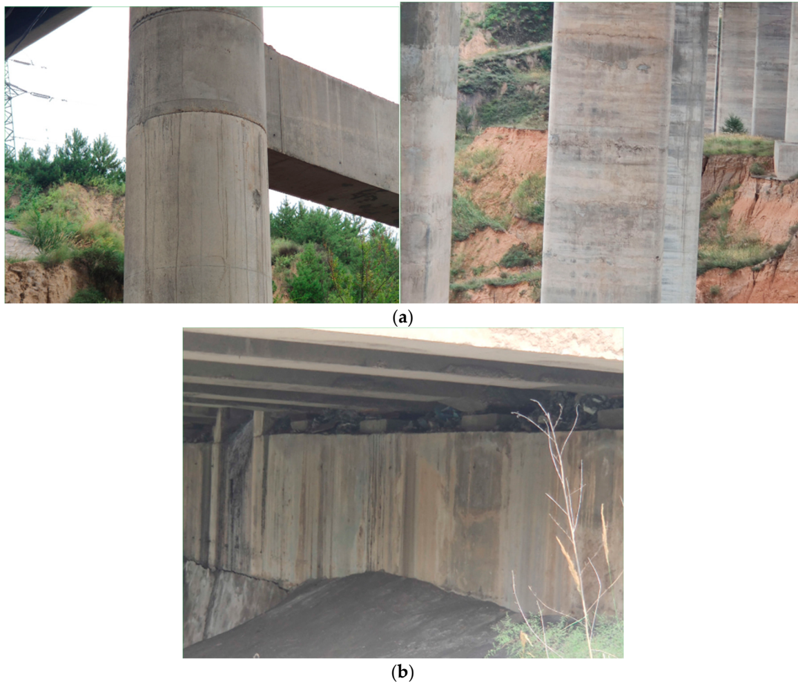
Figure A5. Disease observation of piers and caps: (a) pier body is basically intact; (b) caps are basically intact.
