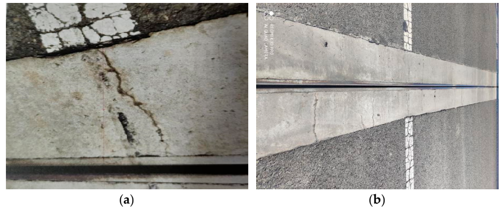
Figure A3. Disease observation of telescopic device: (a) defects in anchorage zone of expansion joint device, slight damage of concrete, cracks, and area of \leq 10\% , scale 2; (b) expansion joint miscellaneous soil filling and cracks caused unevenness, the difference is less than 1 cm, scale 2.
