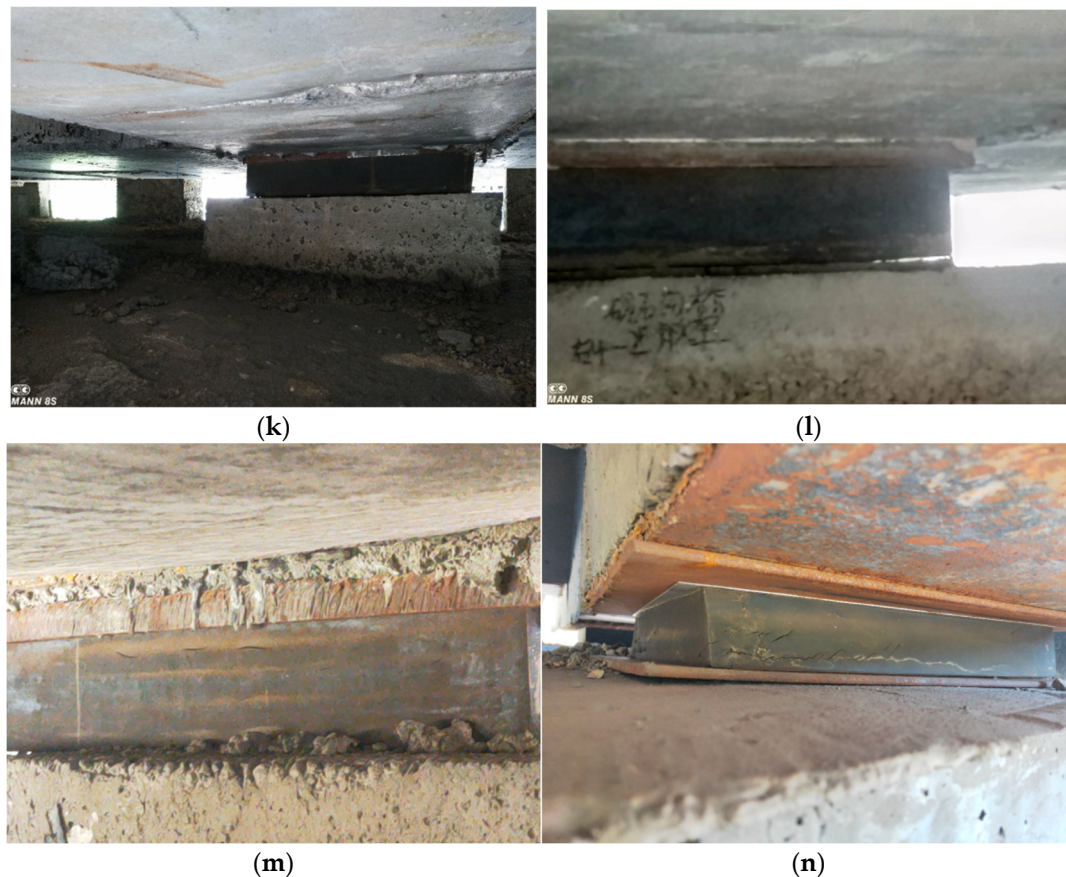
Figure A4. Disease observation of main beam: (a) longitudinal cracks at the bottom of the main girder (a small number of minor cracks in the main girder of <5 mm, the crack width is not exceeded, the single area is \leq 1.0 m 2 , the scale is 2); (b) the spalling angle of the flange plate of the main girder (local concrete spalling, and the single area of \leq 0.5 m 2 scale is 2); (c) main-beam cavity (local concrete holes, and single area \leq 0.5 m 2 scale is 2); (d) honeycomb pockmarked surface at wet joint (there is a large area of honeycomb pockmarked surface, and the cumulative area is less than or equal to 50% of the component area, the scale is 2); (e) spalling-off angle at wet joints (local concrete spalling occurs and the single area is \leq 0.5 square meters, the scale is 2); (f) wet joint seepage (joint-filler leakage and leakage area of >20\% of the whole seam scale is 4); (g) wet seam mesh cracks (single area of mesh cracks of \leq 20\% of component area is 2); (h) diaphragm peeling-off angle (single area \leq 0.5 m 2 scale is 2); (i) diaphragm void hole (local concrete void and single area of \leq 0.5 m 2 scale is 2); (j) diaphragm mesh cracks (mesh crack single area of \leq 1.0 m 2 , scale is 2); (k) left bearing void (void phenomenon appears, scale is 4); (l) right bearing void (void phenomenon, scale of 4); (m,n): bearing aging deterioration, cracking (surface dirt cracks, and the crack length is greater than the corresponding side length of 10%).
