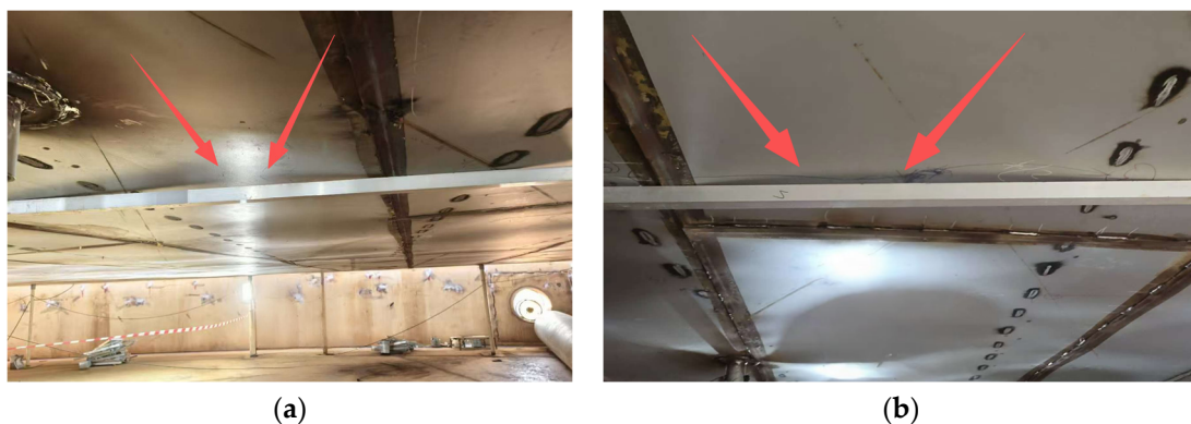
Figure 1. Irregular deformation of the floating roof bottom plate welding measured on-site: (a) irregular deformation in the middle area; (b) irregular deformation in the edge area.
