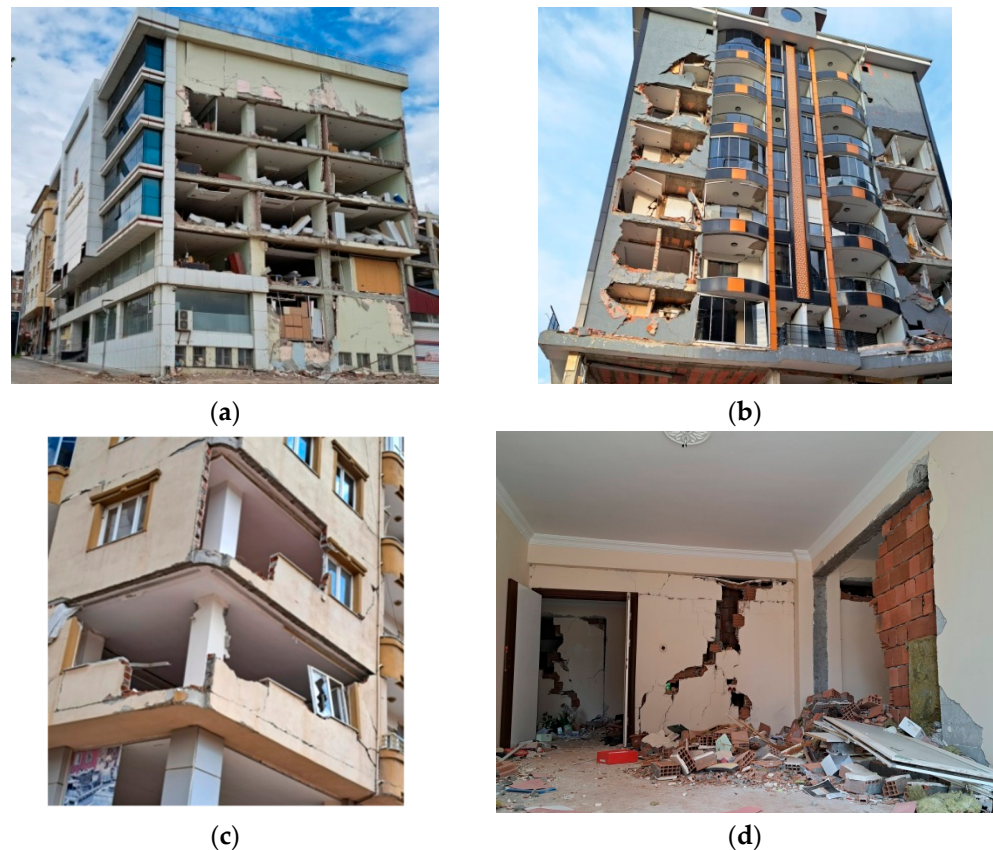
Figure 1. Failure of infills not well encased in the structure: (a,b) infills built exterior to the RC structural elements, (c) exterior infills built between slabs in overhangs, and (d) interior infills with a gap along the infill perimeter and RC members also without connection between the two leaves of bricks.
