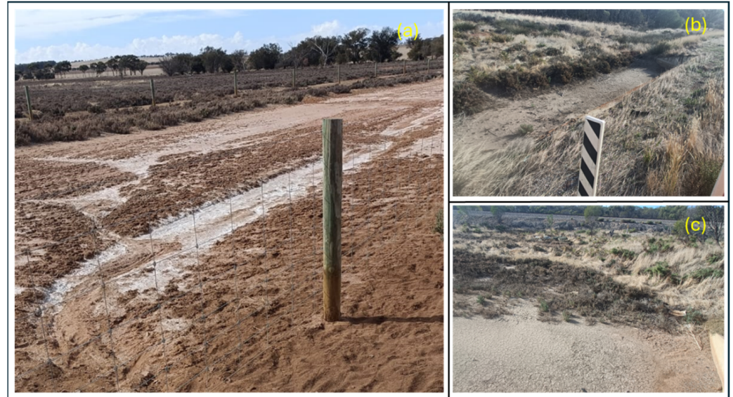
Figure 5. (a) Salt leaching out in culvert vicinity, (b,c) salt tolerant plant (beaded glasswort) in the vicinity of culvert site.
