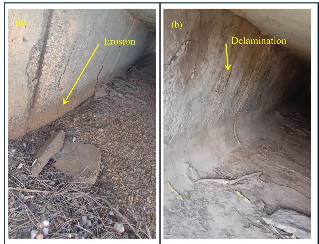
Figure 8. (a,b) Delamination observed in culvert unit.
