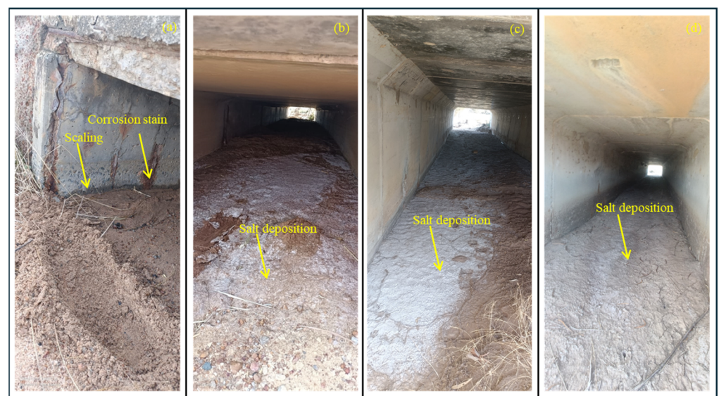
Figure 9. (a) Scaling and corrosion stain in culvert 2, (b–d) evaporated salt deposits on silted soil inside the culverts 3, 13, and 14.
