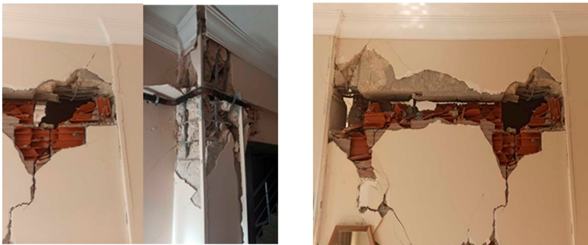
Figure 10. Damage observed in the building.
