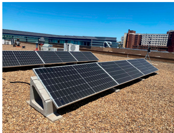
Figure 1. Real PV installation located on the roof of the School of Industrial Engineering of Badajoz (University of Extremadura).
