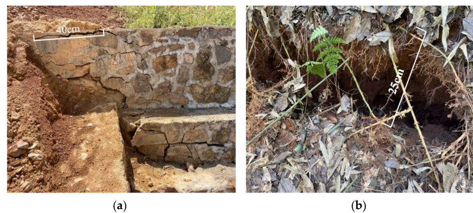
Figure 3. Landslide deformation signs: (a) cracks in the retaining wall at the front edge of the landslide; (b) landslide trailing edge crack.
