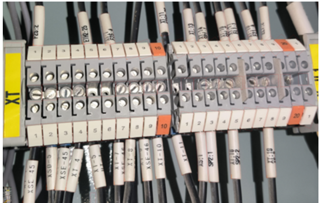
Figure 6. The physical entity of secondary screen cabinet terminal block.
