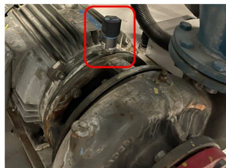
Figure 2. Vibration sensor (in the red square) installed on the motor of a chiller machine.
