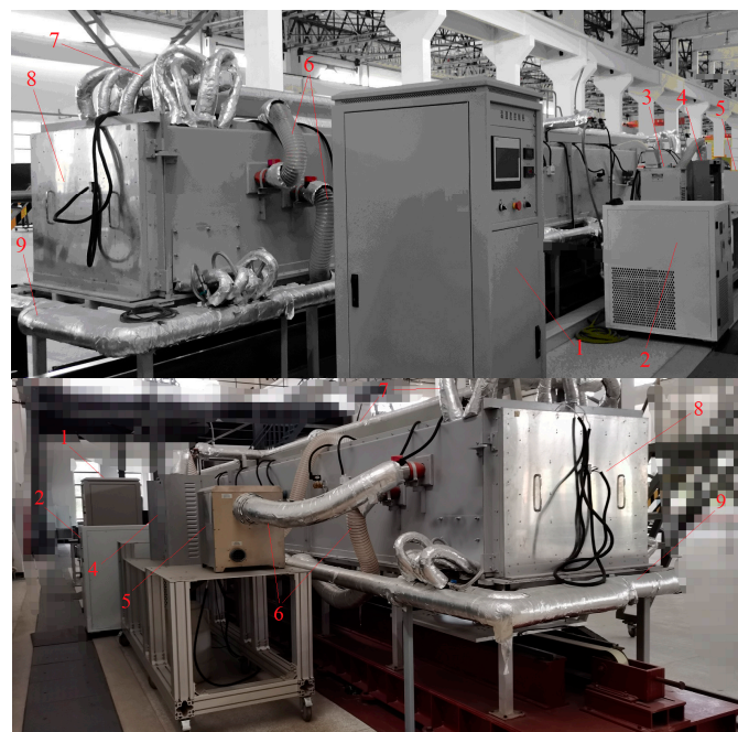
Figure 9. Control cabinet and devices of temperature and humidity control system. 1. Temperature and humidity control cabinet; 2. Constant-temperature water tank; 3. Recirculating heating/refrigerating machine; 4. Humidifier; 5. Recirculating dehumidifier; 6. Humidification/dehumidification steam pipes; 7. Water intake pipes; 8. Enclosed chamber; 9. Water return pipes.
