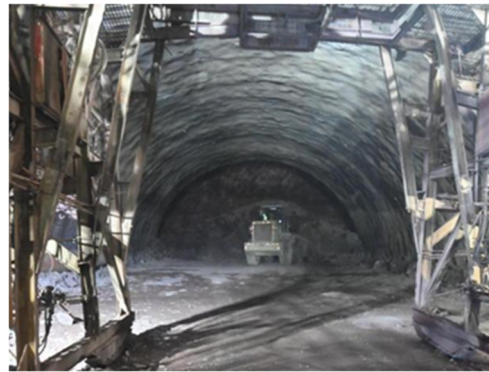
Figure 10. Slagging after tunnel blast.
