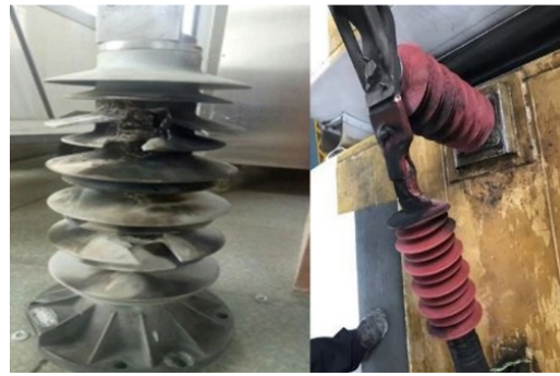
Figure 1. Damage and explosion accidents of high-voltage equipment on electric locomotive.
