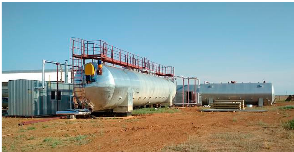
Figure 1. Typical for the Russian Federation block-modular anaerobic bioreactors based on railway tanks (with the permission of SelkhozBioGaz LLC) [39].
